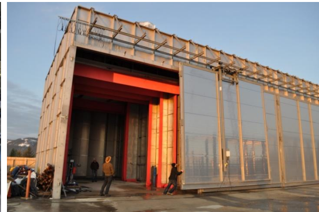
Installation of new drying kilns finalized during Q1 2012 – completed with boilers
